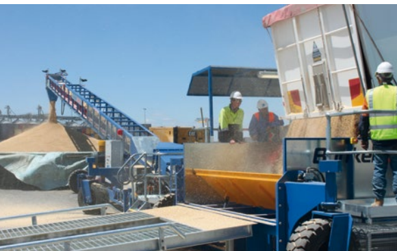
Drive Over Hopper in operation
